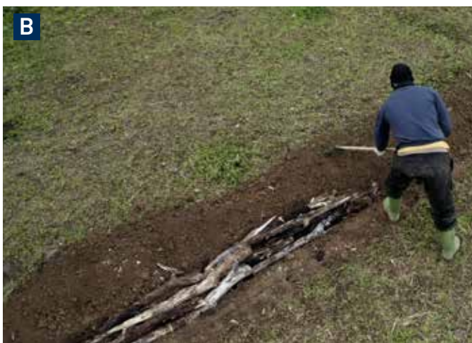
Figure 3. Placing trunk beds in garden crops: A) arrangement of the layer of logs; B) the logs are covered with earth extracted from the trench itself. Photos: AVVideo.
